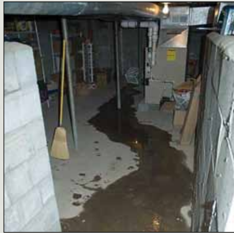
Slab Foundation Leaks (Interior)
