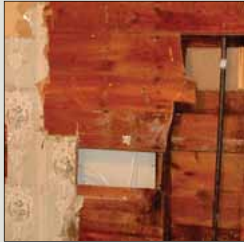
Wall & Ceiling Leaks (Interior)
