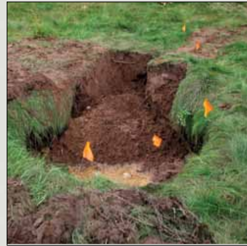
Water Main/Ground Leaks (Exterior)
